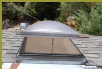
Photo 5. Operable skylights should be closed when a wildfire threatens. Similar to windows, they should incorporate a screen to resist the intrusion of embers (also good for insects!).
