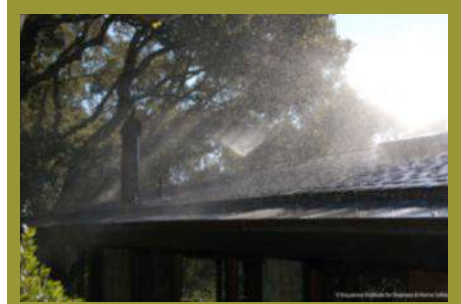
Photo 1. Roof mounted sprinkler.
