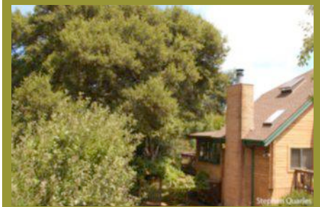
Photo 3. The vulnerability of skylights on a steep-slope roof will depend on the potential for an extended radiant heat exposure to the roof and skylight unit.
